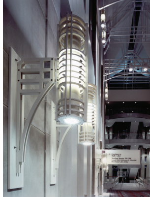
Custom lighting fixtures – Philadelphia Convention Center
